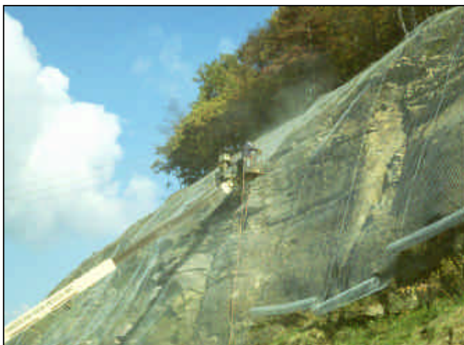
Example of Rockfall protection netting
