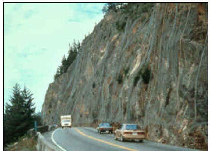
Example of Rockfall protection netting
